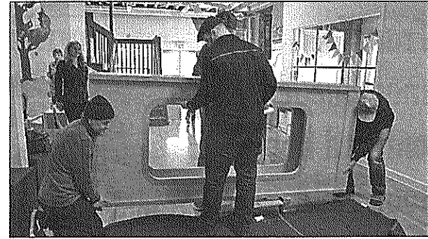
Adrian French (left), COSI manager of exhibit fabrications, teams up with (left to right) Steve Haberichter, Carson Slager and Jim Elliott to install a display case at KidsWork Children's Museum. NURIA MATHOG/22ND CENTURY MEDIA
